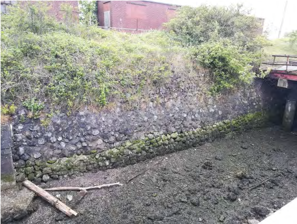
Plate 9.1 The intertidal area to the south of the existing pier structure near the pumping station, showing poor quality of habitat and limited colonisation and species diversity.
