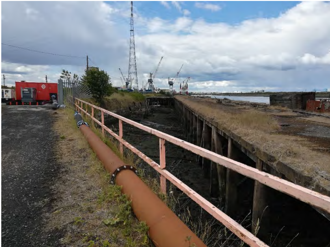
Plate 9.2 The existing South Bank Wharf to be demolished, with the pumping station on the left. Minimal colonisation of the pillars supporting the deck of the wharf is evident.
